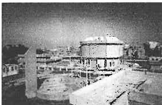
Waste Water Project, Cairo Infrastructure to treat and collect sewage.
