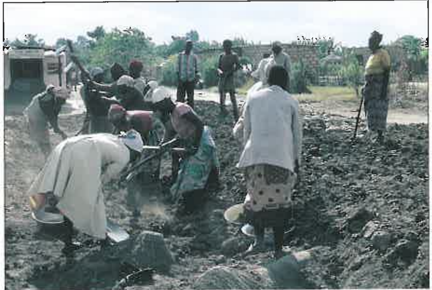
The Federation of Norwegian Cooperative Building and Housing Associations (NBBL) is engaged in development assistance, and has contributed to development and improvement of Bauleni a part of Lusaka, Zambia. (Photo: NBBL)
